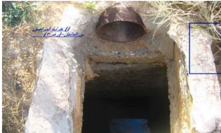
Fig. 8 Rainwater in sub-surface reservoirs "Haraba"
